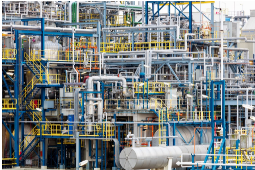
Figure: Industrial pipe network, https://www.steeljrv.com/
